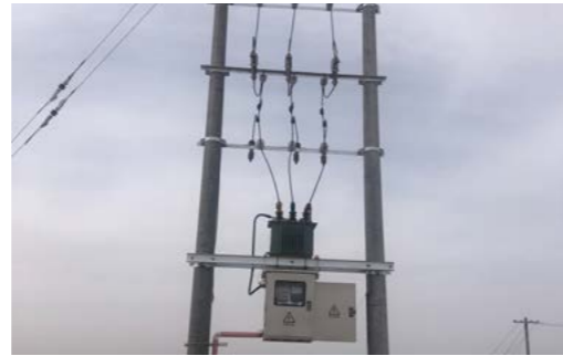
Power facilities after upgrading
